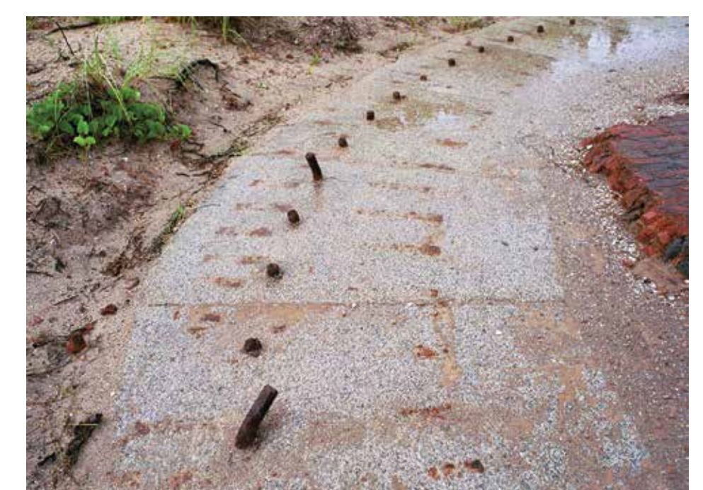
Bolts that held the iron Lighthouse to the granite foundation can be seen
